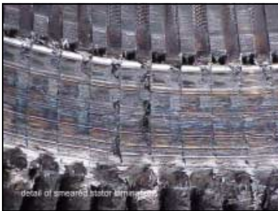
Figure 20. Major mechanical damage to the stator bore; not repairable unless the core is restacked or replaced.
