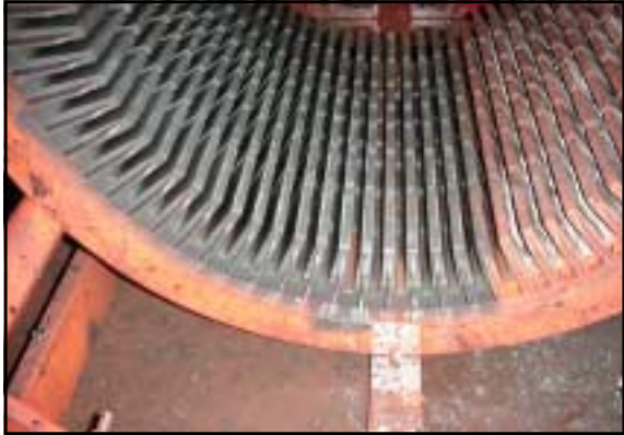
Figure 24. This core has been partially cleaned by using a high-pressure washer to remove the slot insulation debris.
